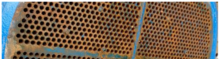
18 Months of use shows virtually no biofouling in the exchange tubes
